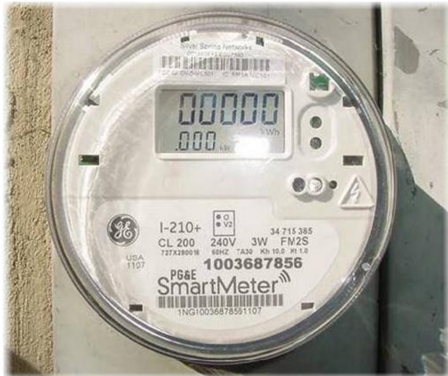
Figure 2.1: A smart meter installed on the electric main.
