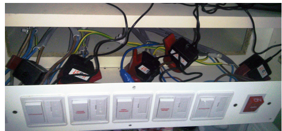
Figure 2.6: CT clamps installed on individual kitchen appliance power cables
